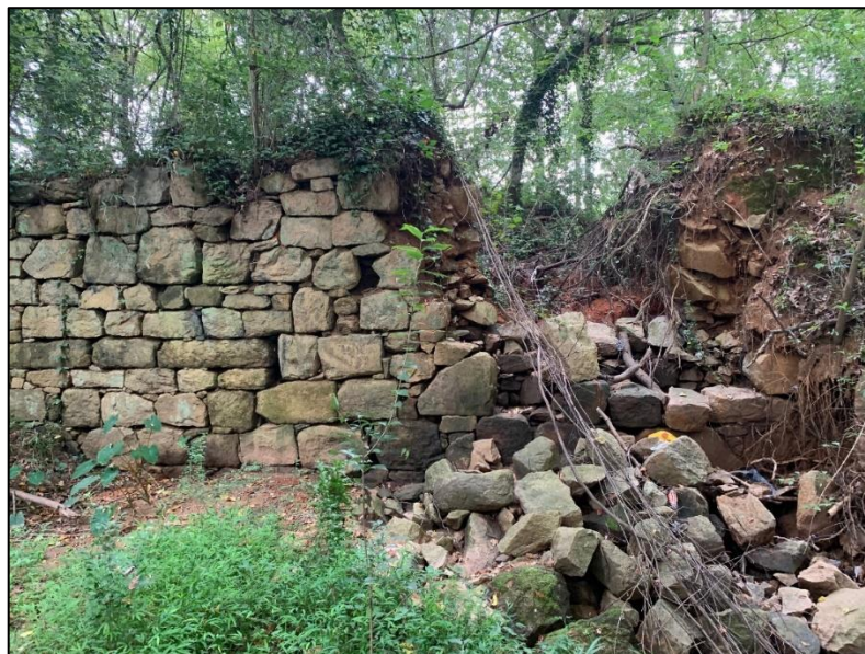
Erosion of existing historic wall to be prevented by project
