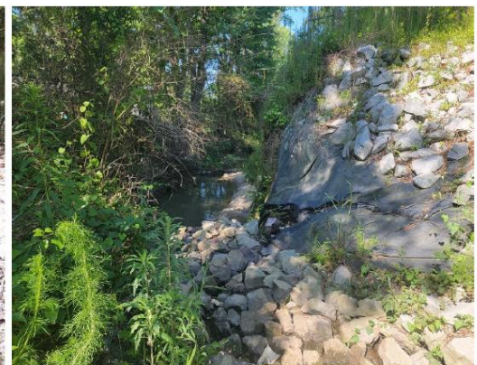
Failed bank stabilization with riprap
